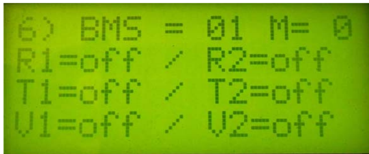
Fig. 8. Menu 6: the state of the BMS inputs and outputs 1/2.
